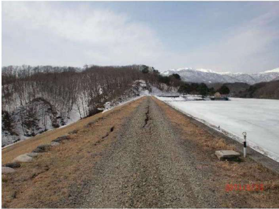
Figure 11. Nishigo Dam; cracking on the crest
